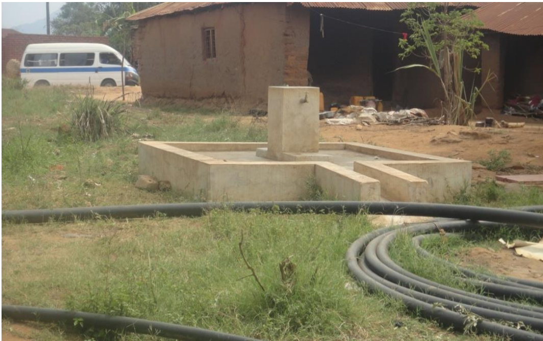
Figure 4.6: Community managed piped water point
