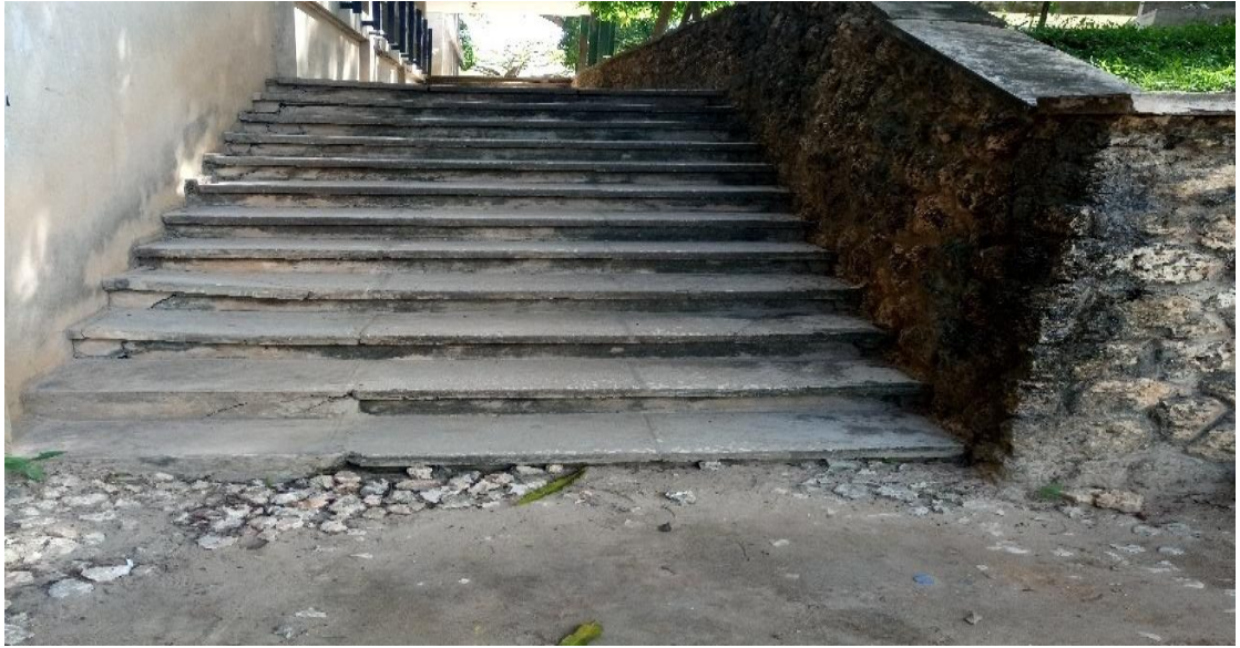
Plate 4.10: Unsupportive building structures for VIS at UDSM
