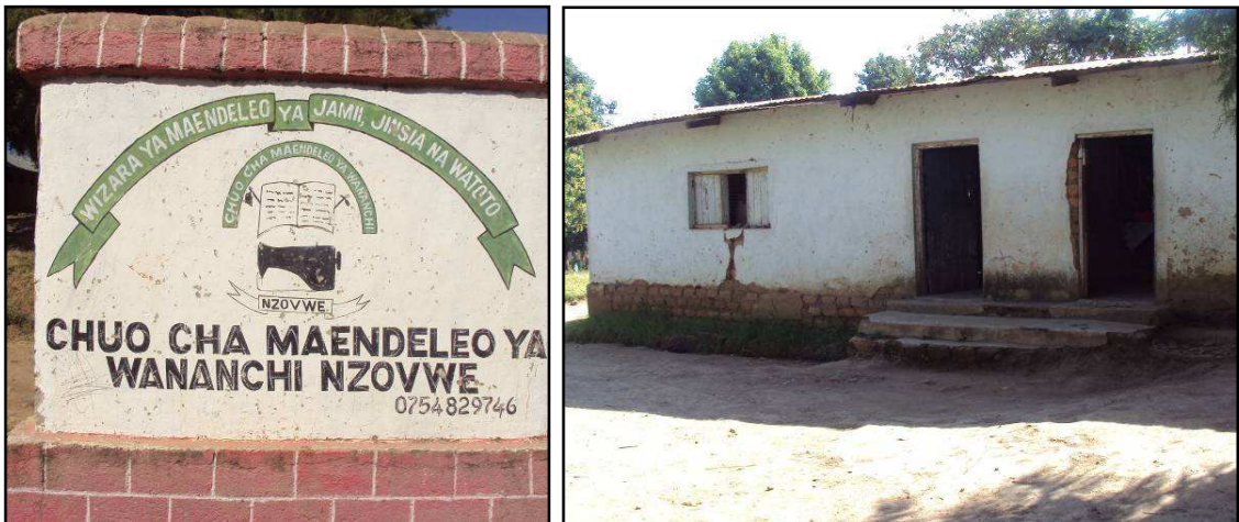
Figure 4.3: Poor Infrastructure as a Challenge Facing FDCs
