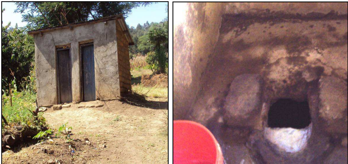
Figure 4.2: Poor infrastructure within FDCs
