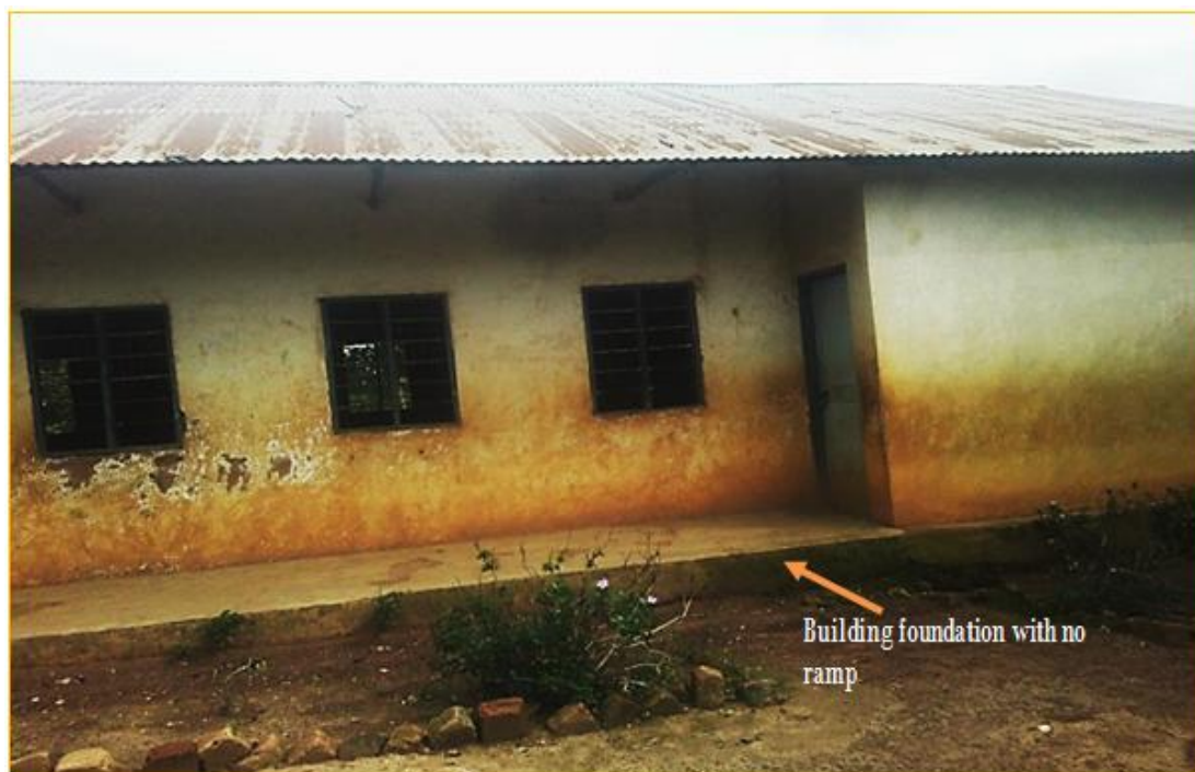
Figure 4.5 A Classroom and office which has no ramp
