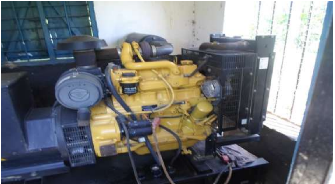
Figure 4.6: Generator for water pumping in Dalla village
