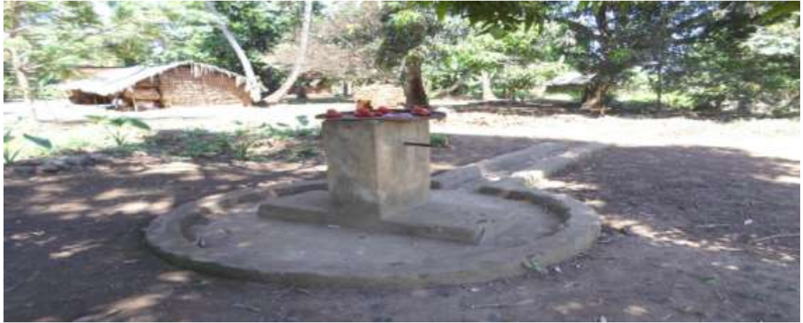
Figure 4.5: Water point in Dalla village after project
