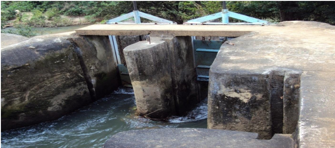
Figure 6.2: Intake facility with control devices in MIS
