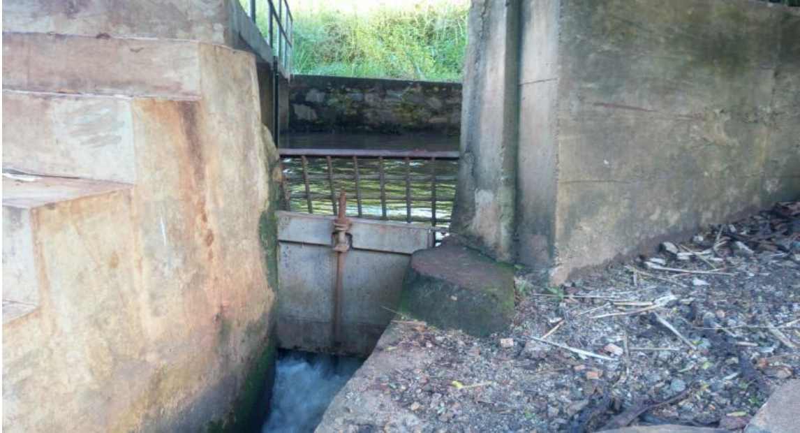
Figure 6.3 Intake facility with control devices in KIS
