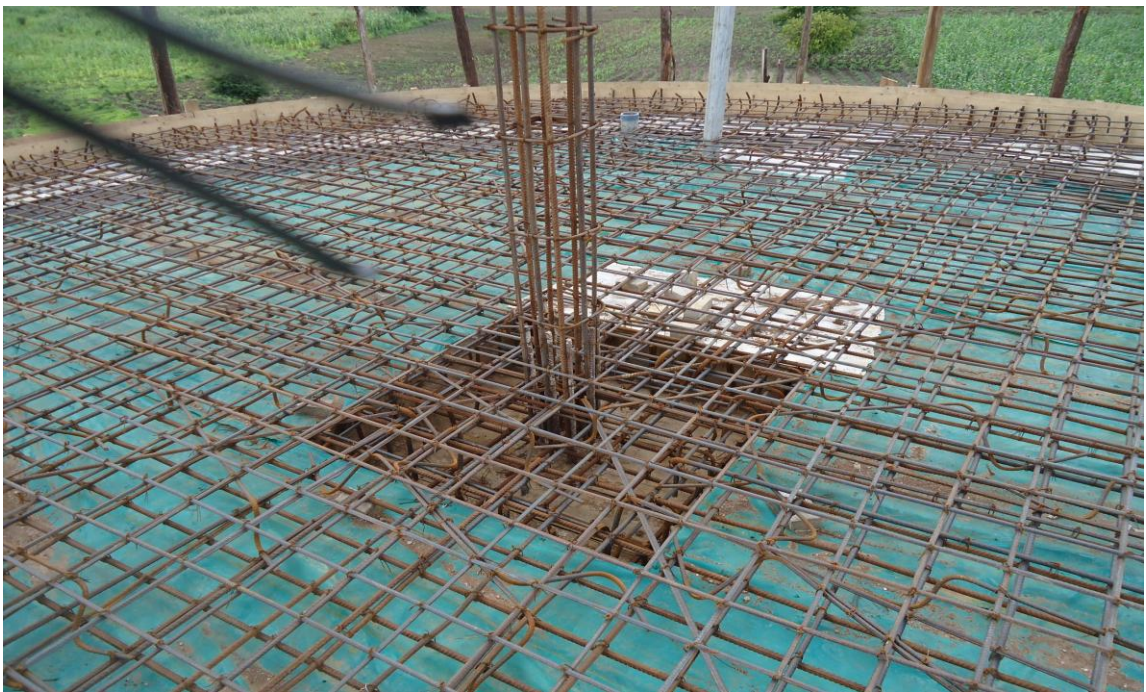
Figure 3: The closeness of iron bars setting for construction of water tank base on top of water tower at Segese village. This photo reflects that there is a daily close supervision from the consultant because; A Consultant having sufficient time to supervise a works projects when compared to in – house staff.
