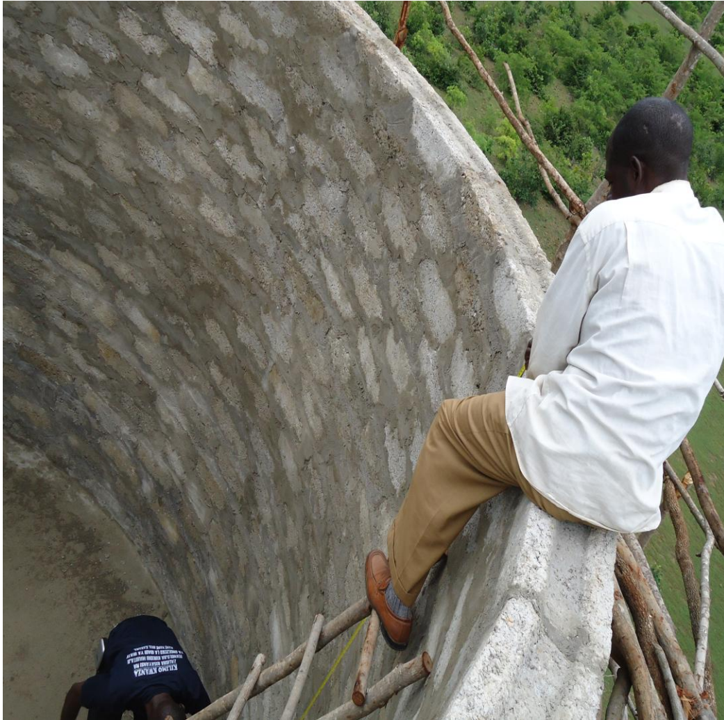
Figure 2: The Client representative makes verification of the height of Water Tank at Chela village. He is receiving information from Consultant Technician (on top). The Client representative observed that the height stated is exactly right to what constructed measurement was, it's due to close supervision from the Consultant. The height of water tank justifies the capacity of water tank; the task of the consultant is to make sure the height stated on BOQ must be constructed exactly in order to satisfy the need expected. The photo shows Client representative verify the height of the water tank from the consultant supervisor.
