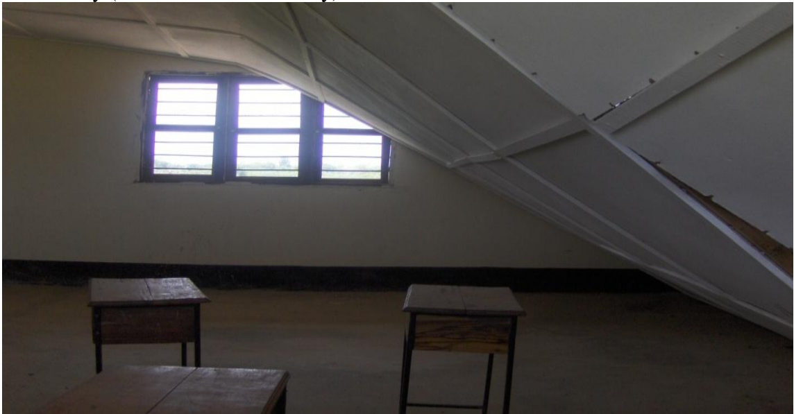
Figure 4: This is the broken ceiling board at Bulyang'hulu Secondary School. This is a result of poor supervision on construction by in-house staff.
