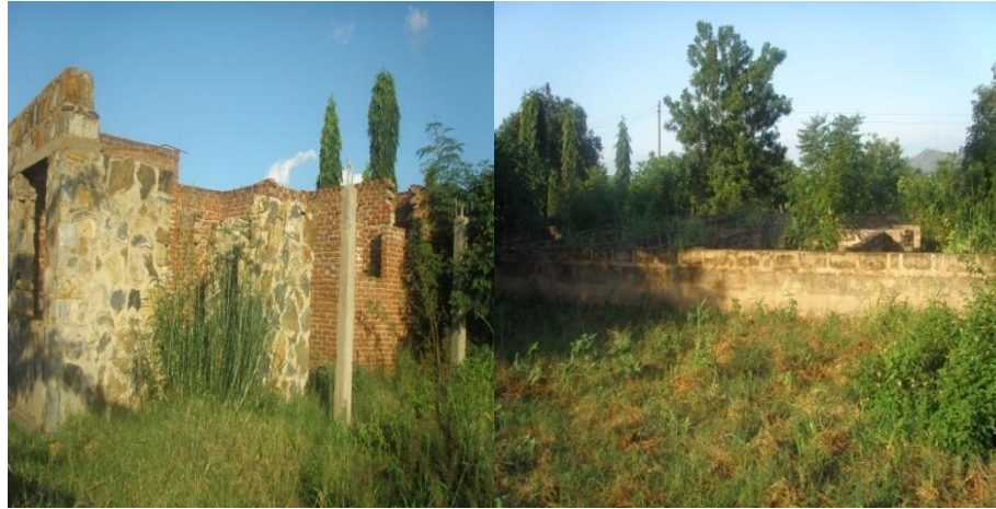
Figure 4.5: Abandoned Incomplete Buildings at Mlimakola Area
