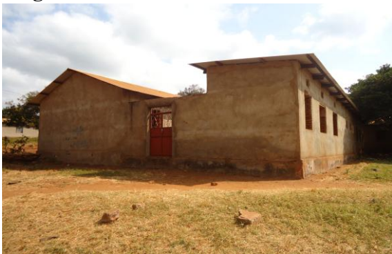
Plate 2: Delayed Teachers house building at Kwaang'w Secondary School since 2007 at Kiongozi village
